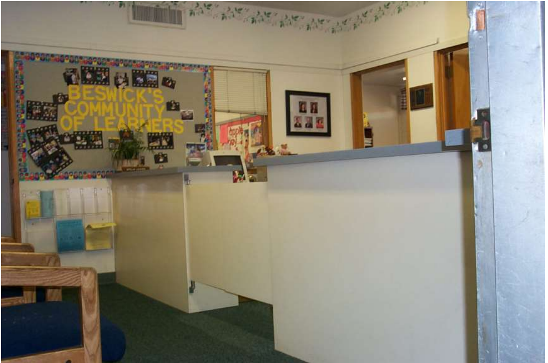
Disabled Counter Access Needed (ADA) – Beswick Elementary School
