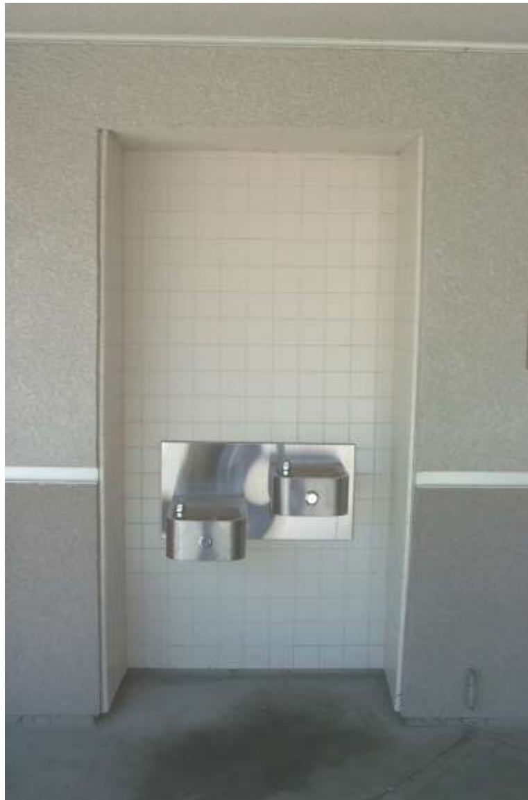
Accessible Drinking Fountains – Ladera Elementary School
