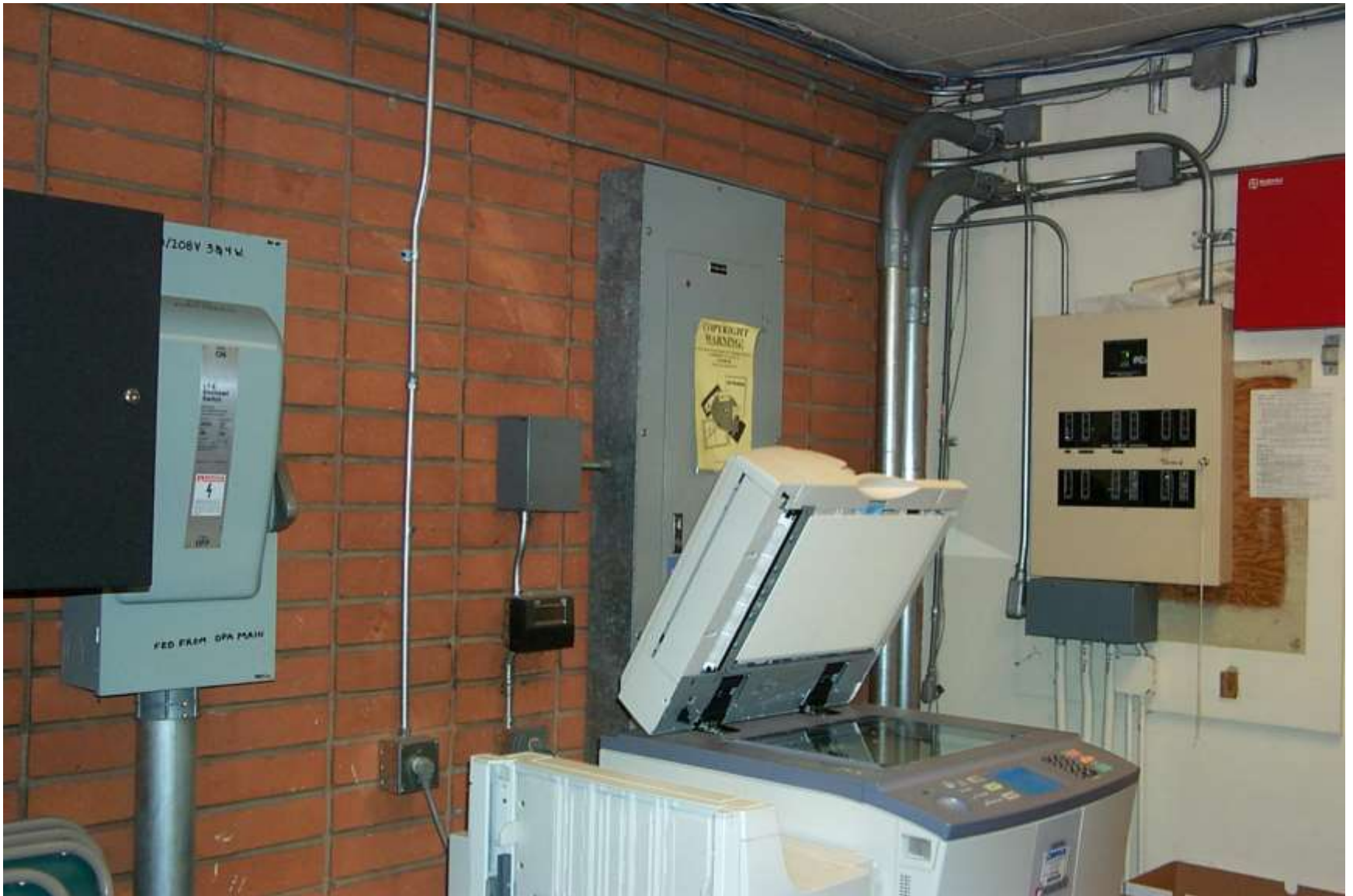
Power/Data/Fire Alarm/Bells/Intercommunication Systems Needs – Beswick E.S.
