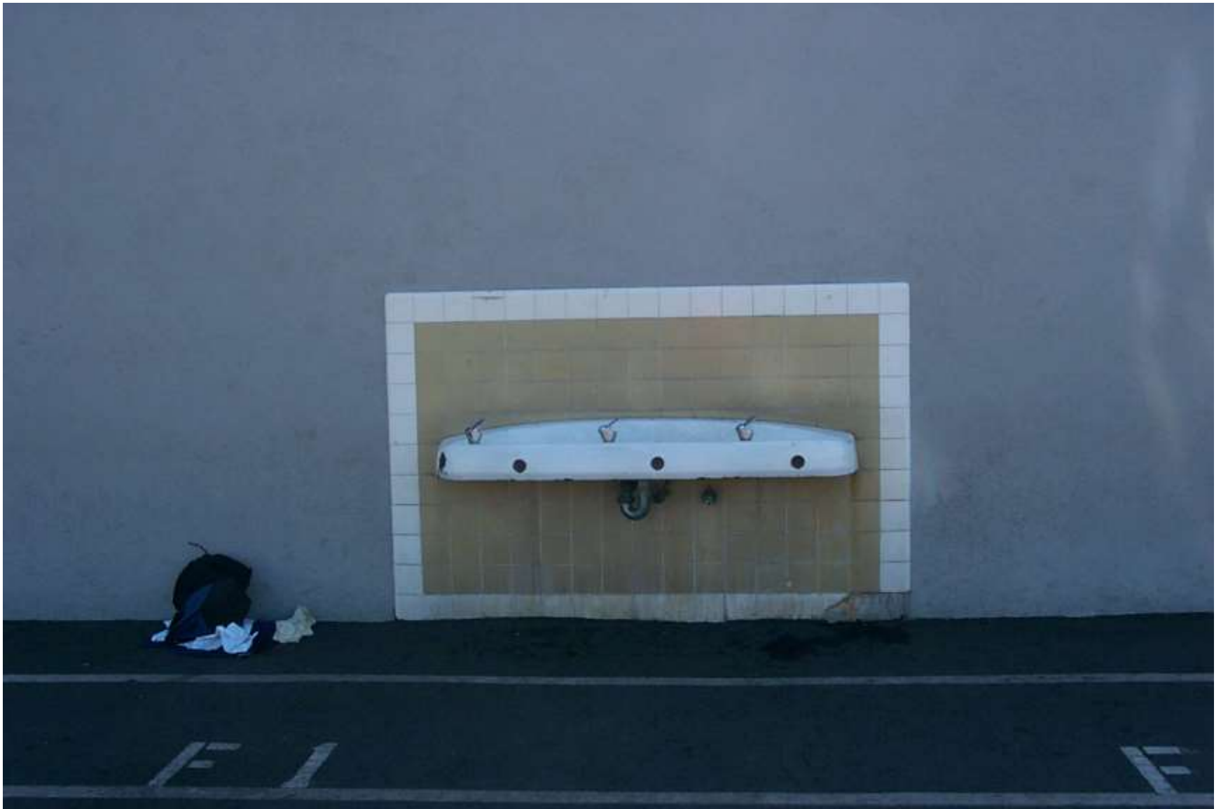
Disabled Access – Drinking Fountains – Beswick Elementary School
