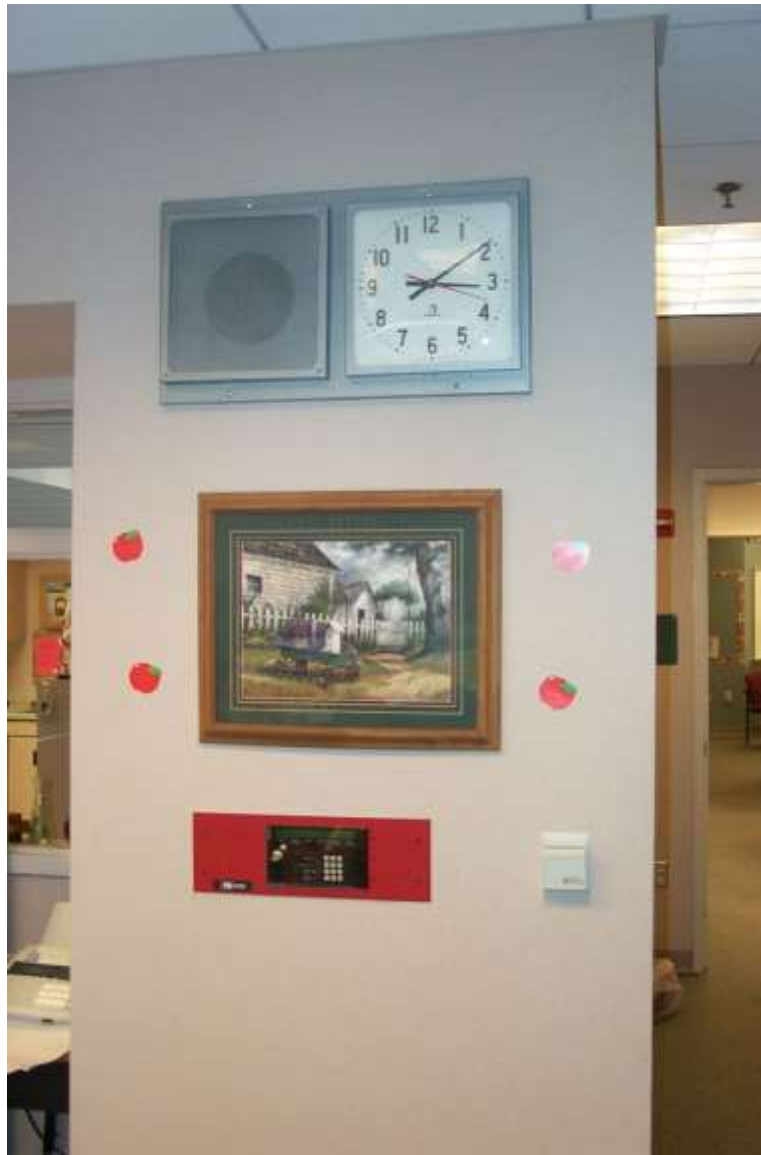
Fire Alarm Panel, Communications Outlet – Myford Elementary School
