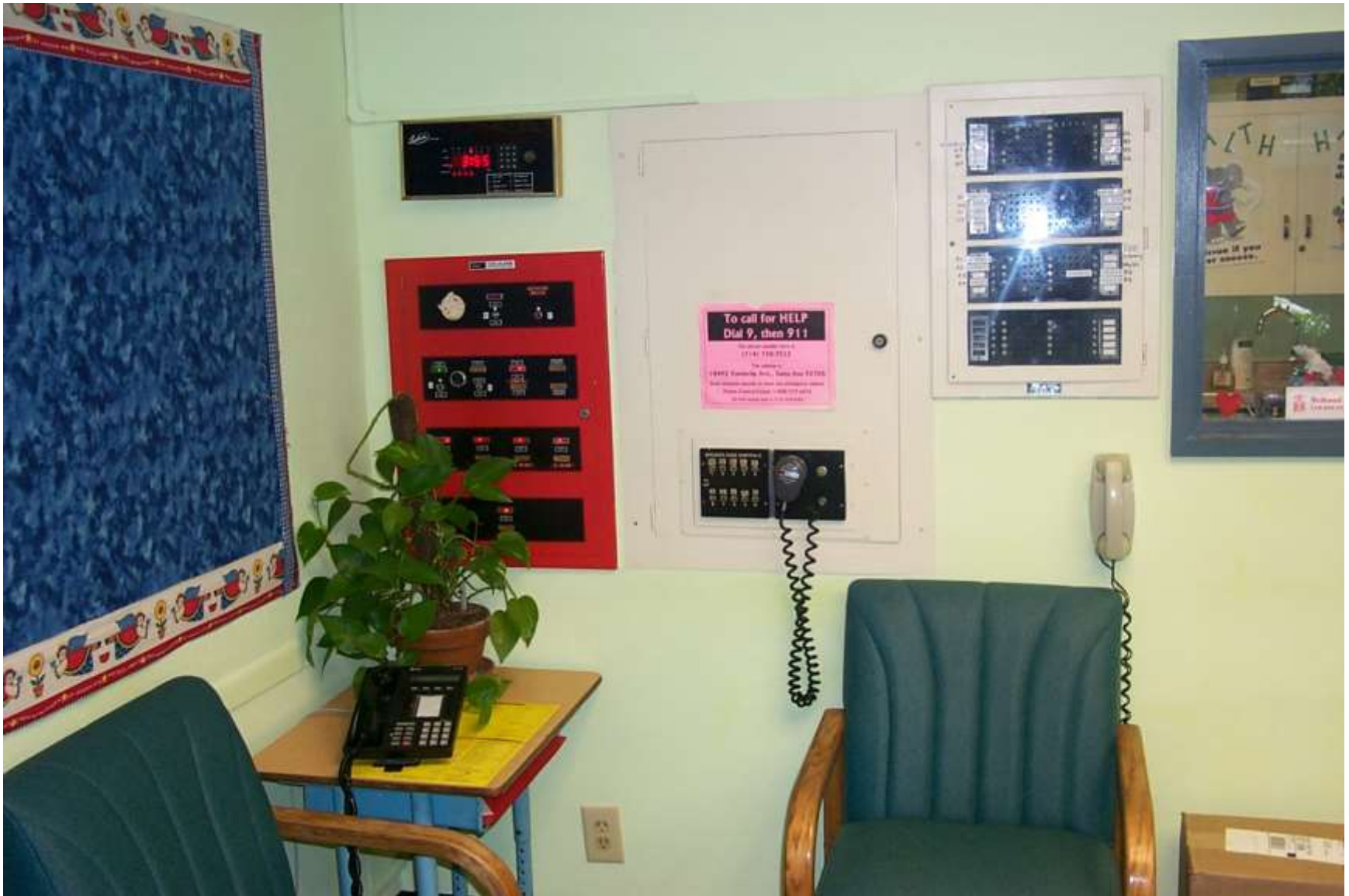
Life Safety Communications System – Guin Foss Elementary School
