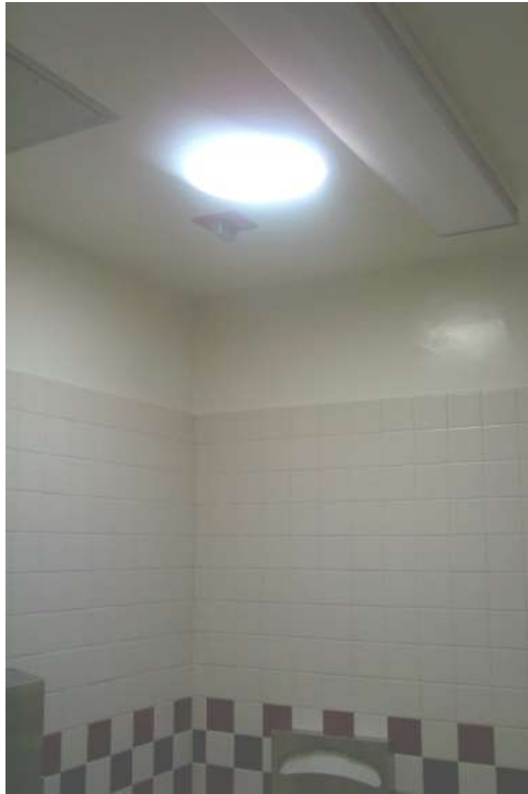
Solatube Skylights for Energy Savings – Hewes Middle School
