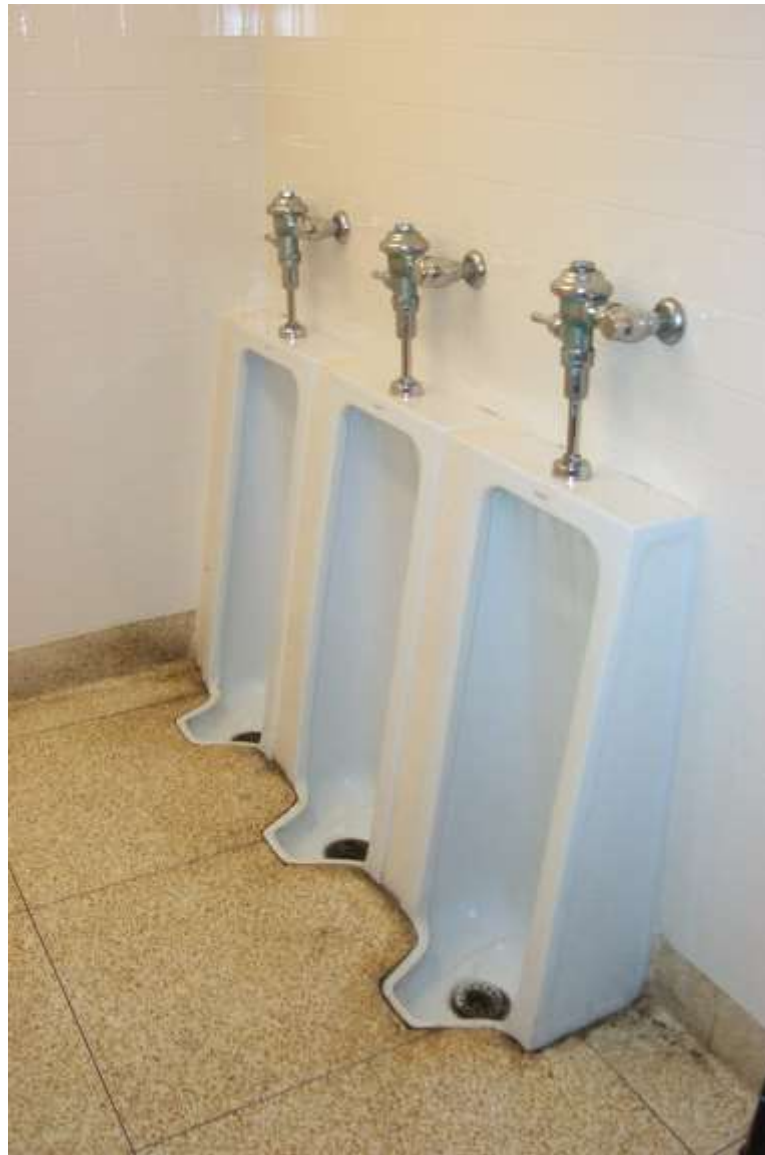
Restroom Renovation Needed (ADA) – Foothill High School
