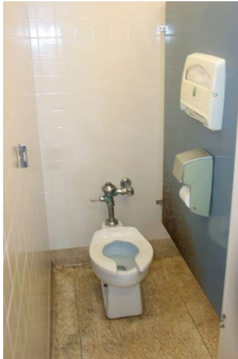
Restroom Renovation Needed – Foothill High School
