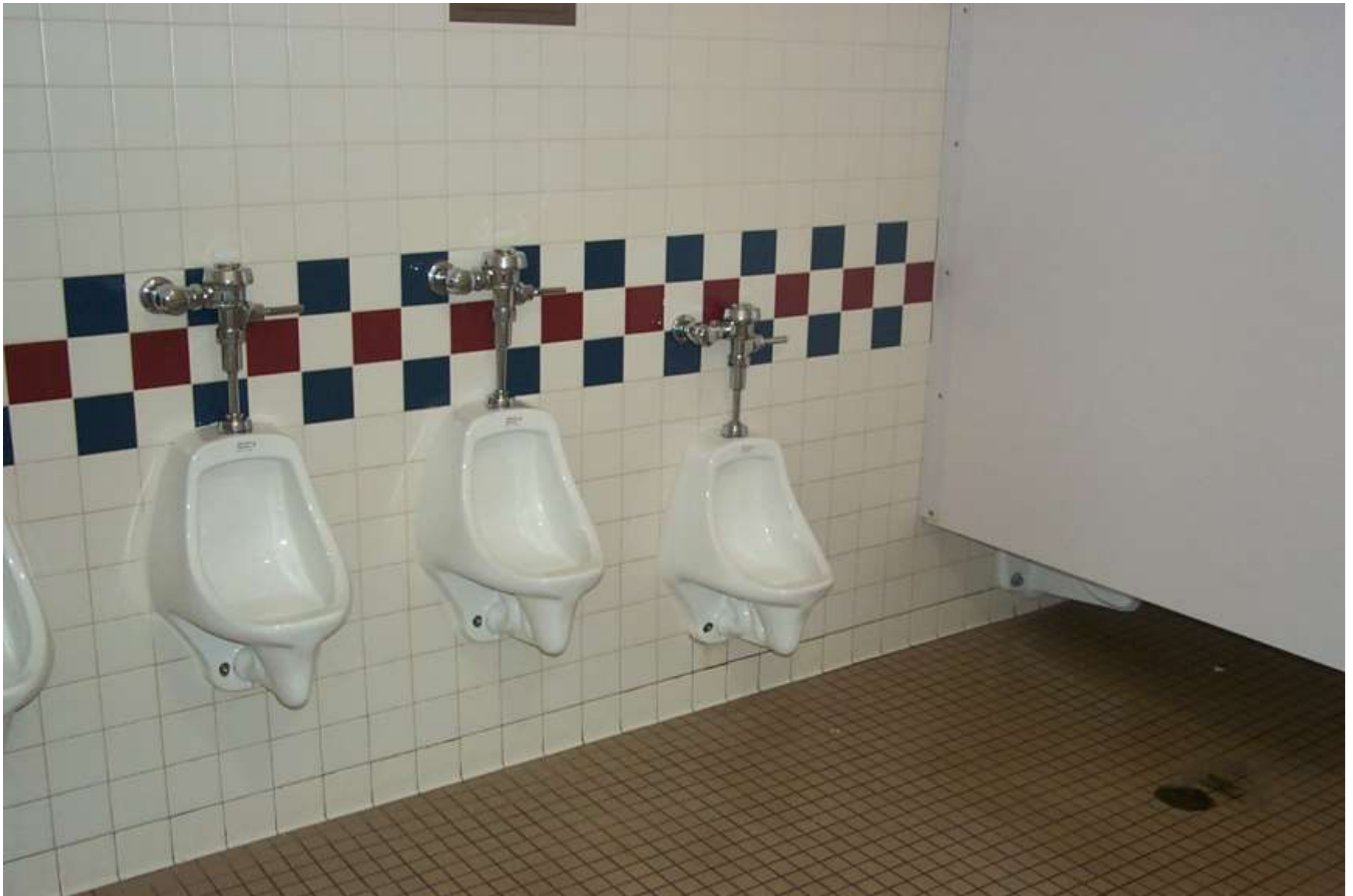
Accessible Restroom – Hewes Middle School
